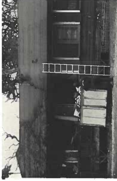
The Maui Community Correction Center crew prepares to cut the burned building in-half to save the unburned portion.
