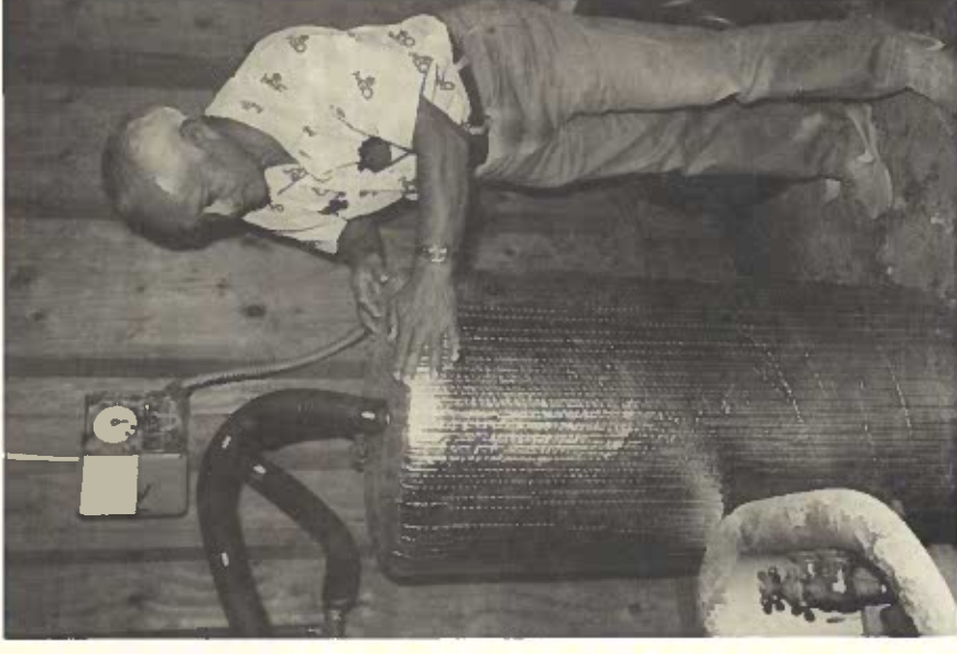
Fred Baisa expertly installs a blanket on a water heater under the WAP Program.
