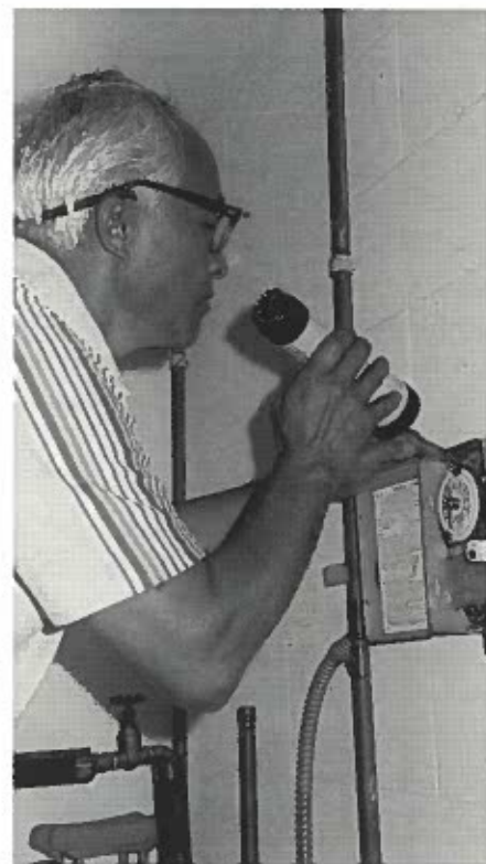
Energy Educator, Fred Basia checks the control panels on a heater.
