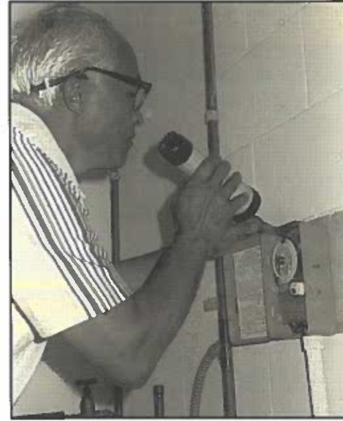
Fred inspects a control panel.
